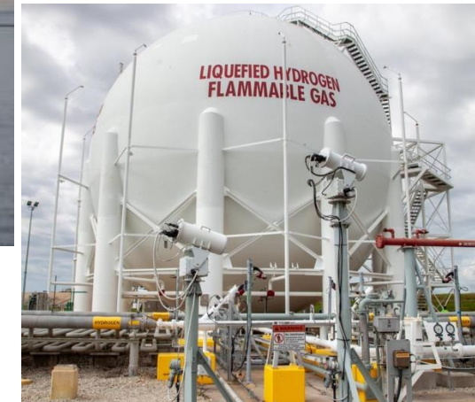
Liquefied H 2 tank at Kennedy NASA space center
